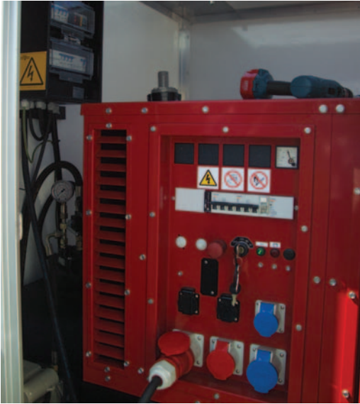
Electrical generator inside B-10
